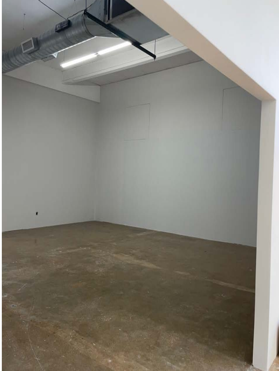
Looking in towards north/east walls from Lobby – note east windows COVERED HERE – slight outlines visible
